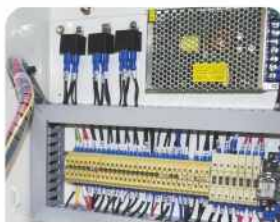
Terminal box inside
